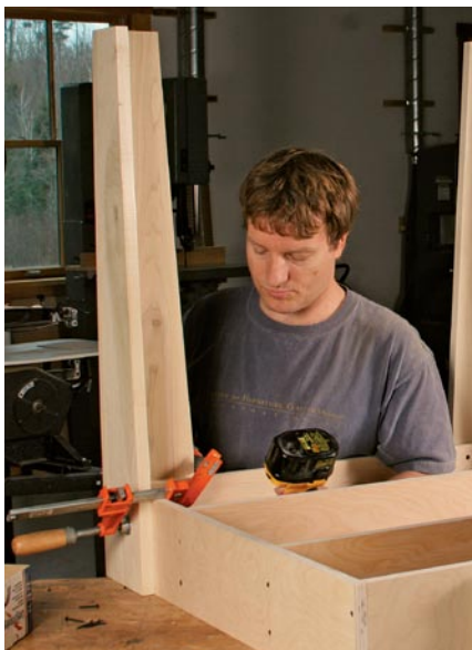
Attach the legs. Glue and clamp the legs in place before screwing them to the base from the inside.
